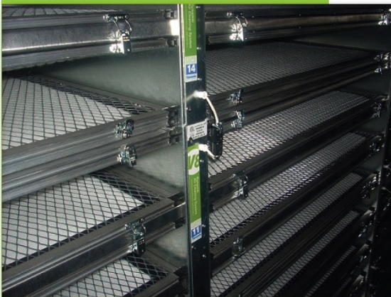
Dynamic V8s in a custom air handler
